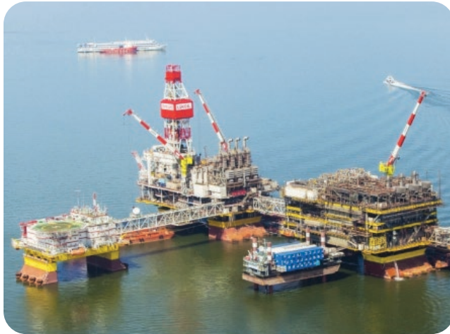
Filanovsky marine ice-resistant stationary platform. Fire cabinets, foam concentrate proportioning system. Customer: LUKOIL
