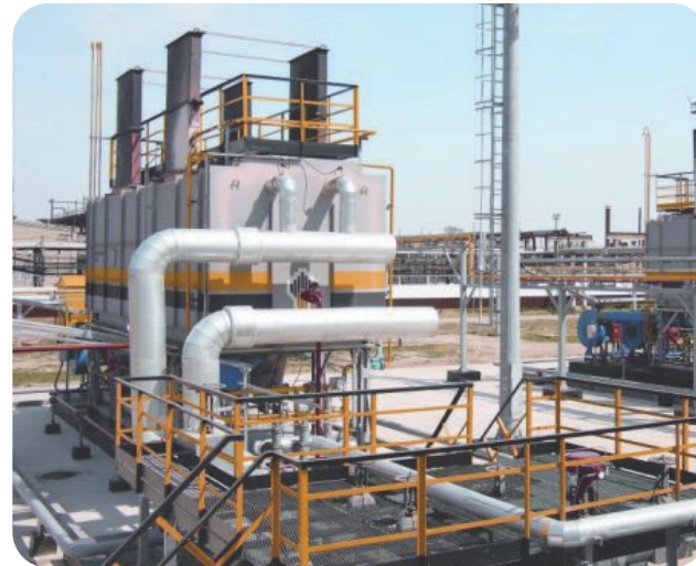
Stavropolneftegaz. Fire extinguishing station, firefighting equipment. Customer: RN - Stavropolneftegaz
