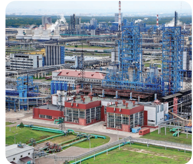
The Ethylene plant. Block container for fire suppression, fire equipment. Customer: KazanOrgSintez
