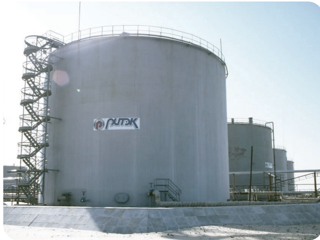
Sandibinsky field tank farm. Foam fire extinguishing installations, firefighting equipment. Customer: LUKOM-A TECHNICAL CENTER (RITEK, LUKOIL)
