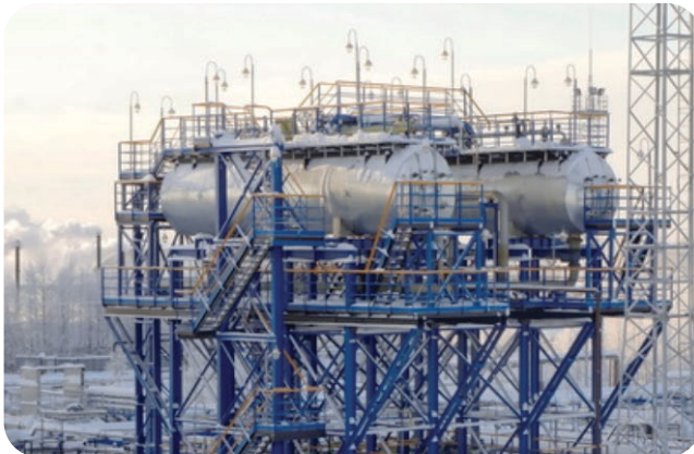
Ukhta Oil Refinery. Block container for fire suppression, firefighting equipment. Customer: LUKOIL-Ukhtaneftepererabotka
