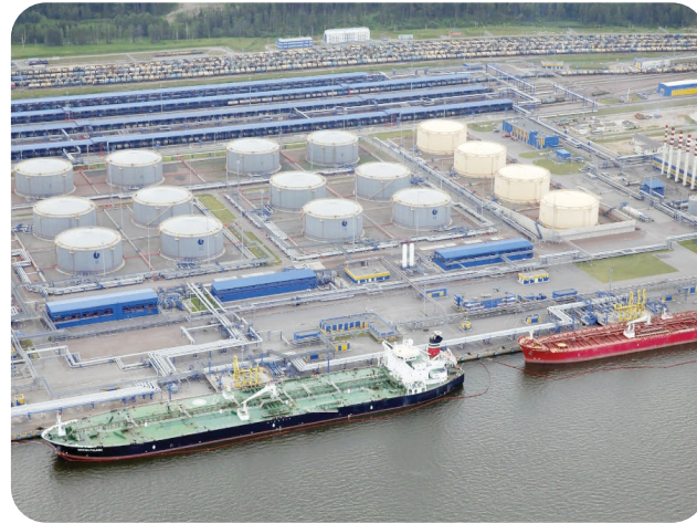
Marine terminal NOVATEK Ust-Luga. Proportioning system, foam generators, fire monitors, fire towers. Customer: NOVATEK
